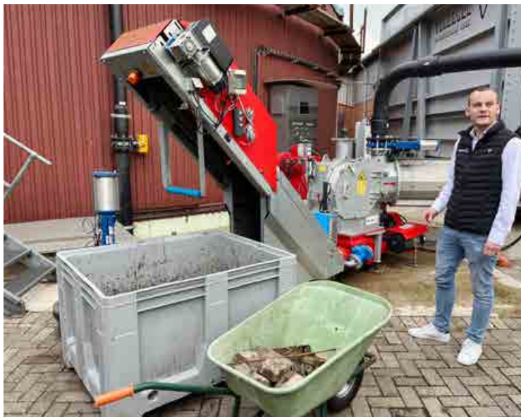
The PreMix ICC in use at the Lamping biogas plant
